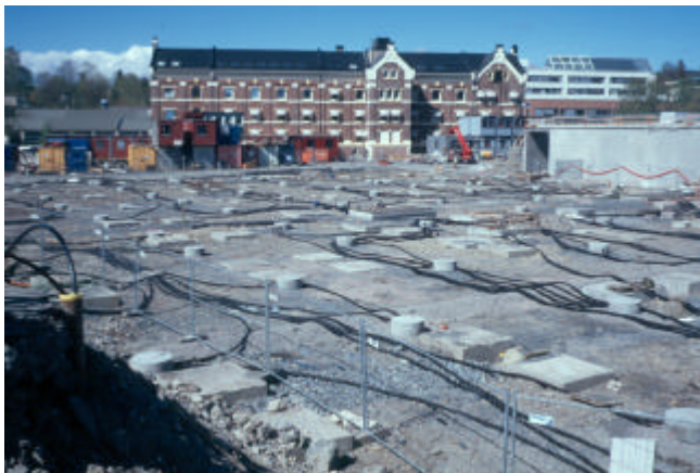
Photo 4. The well field for the Nydalen GSHP in Oslo, Norway; the station will supply several buildings.
