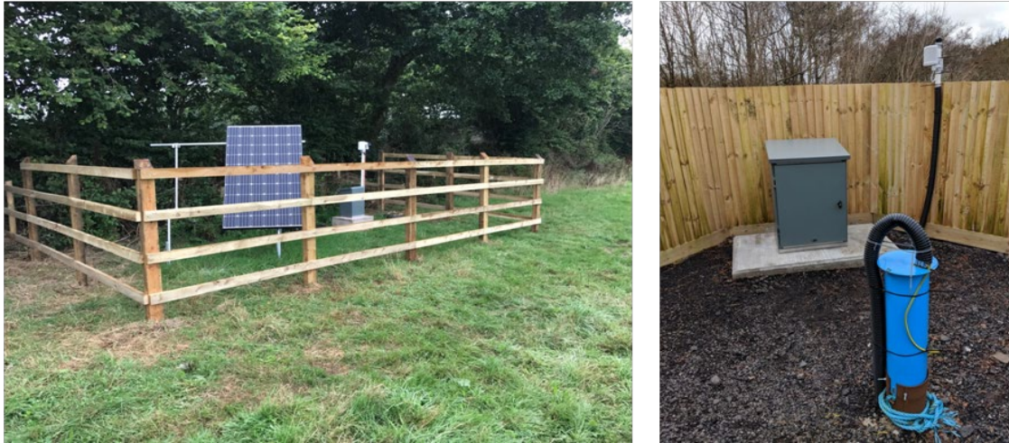
Figure 3: Photographs of two UDDGP microseismic stations. A) a broad-band seismometer station powered by 12V deep-cycle batteries, with continuous recharging via solar-panels. B) a borehole geophone station using mains power and backup batteries. The wellhead standpipe is blue and the black conduit carries the geophone cable underground into the instrumentation cabinet.
